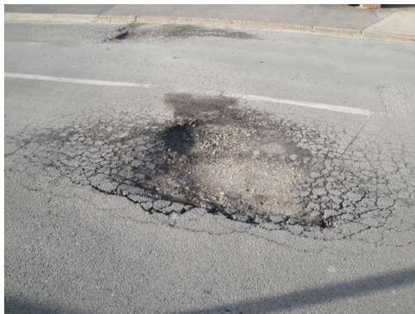
FIGURE 13.14 Thermal stress contributes to the formation of potholes. (credit: Editor5807, Wikimedia Commons)
