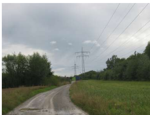
FIGURE 24.9 This high-voltage traction power line running to Eutingen Railway Substation in Germany radiates electromagnetic waves with very long wavelengths. (credit: Zonk43, Wikimedia Commons)
